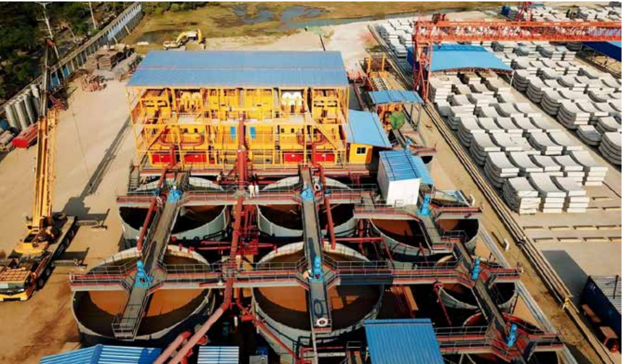
Slurry treatment plant
