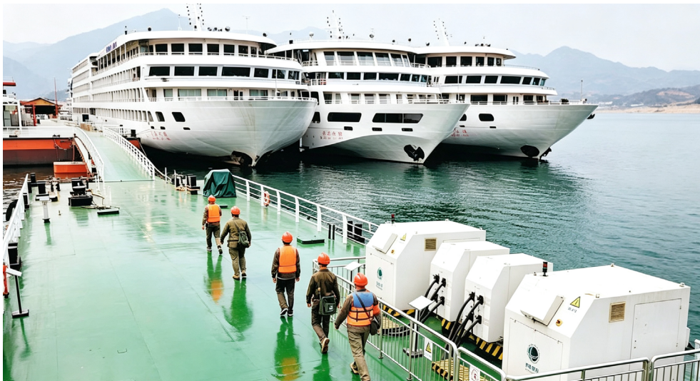
Shore power at the wharves on the Hubei section of the Yangtze River
